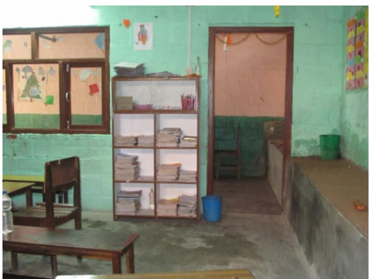
The kindergarten classes are badly in need of paint and repair of the many leaks.
